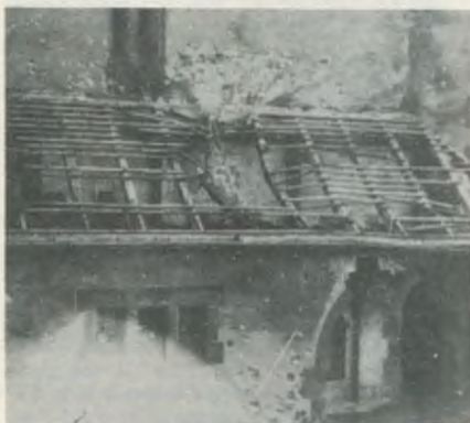
Battered and burned north end of Lutheran church in Philippsbourg. Snapshot was taken in summer of 1945. Vestry in church was used at 275th 1st Bn aid station until the morning of 4 Jan 45, when it was evacuated.
